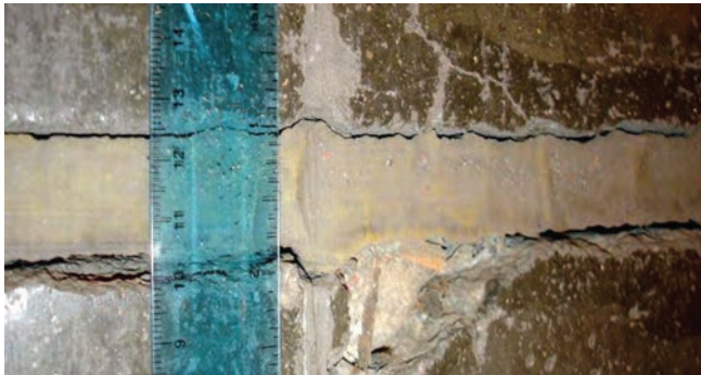
If joint filler has dropped below the floor surface or was not flush originally, joint edge spalling may occur.
