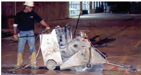
Traditional “wet cut” saws require sufficient slab cure to support the saw’s weight.
