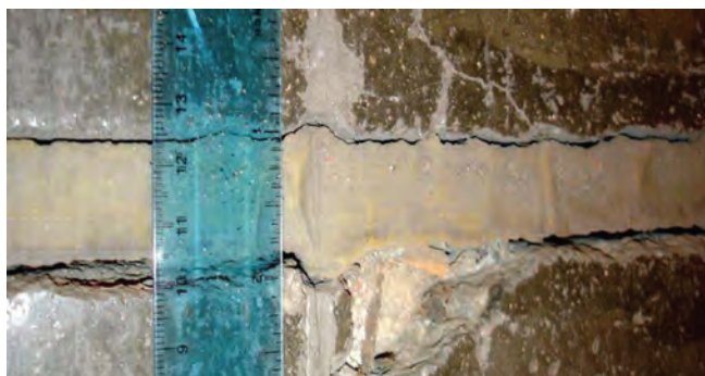
If joint filler has dropped below the floor surface or was not flush originally, joint edge spalling may occur.
