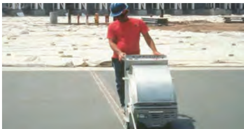
“Early entry” saws allow for joint cutting to be performed within hours of slab placement, reducing the potential of random cracking and allowing for a shallower joint depth to induce cracking below the joint.
