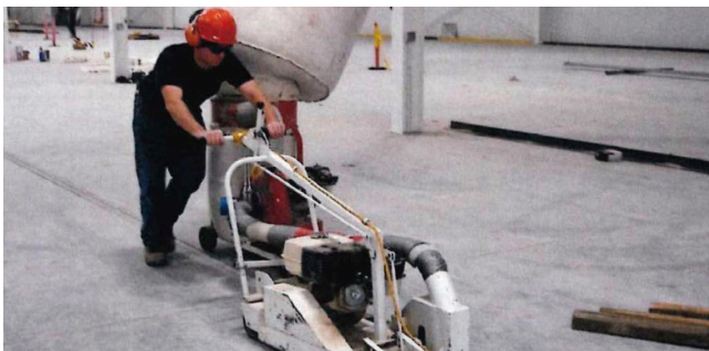
Above: Joints should be cleaned mechanically using a saw (preferably dustless) equipped with diamond or abrasive blade to expose clean, bare concrete along joint walls.
